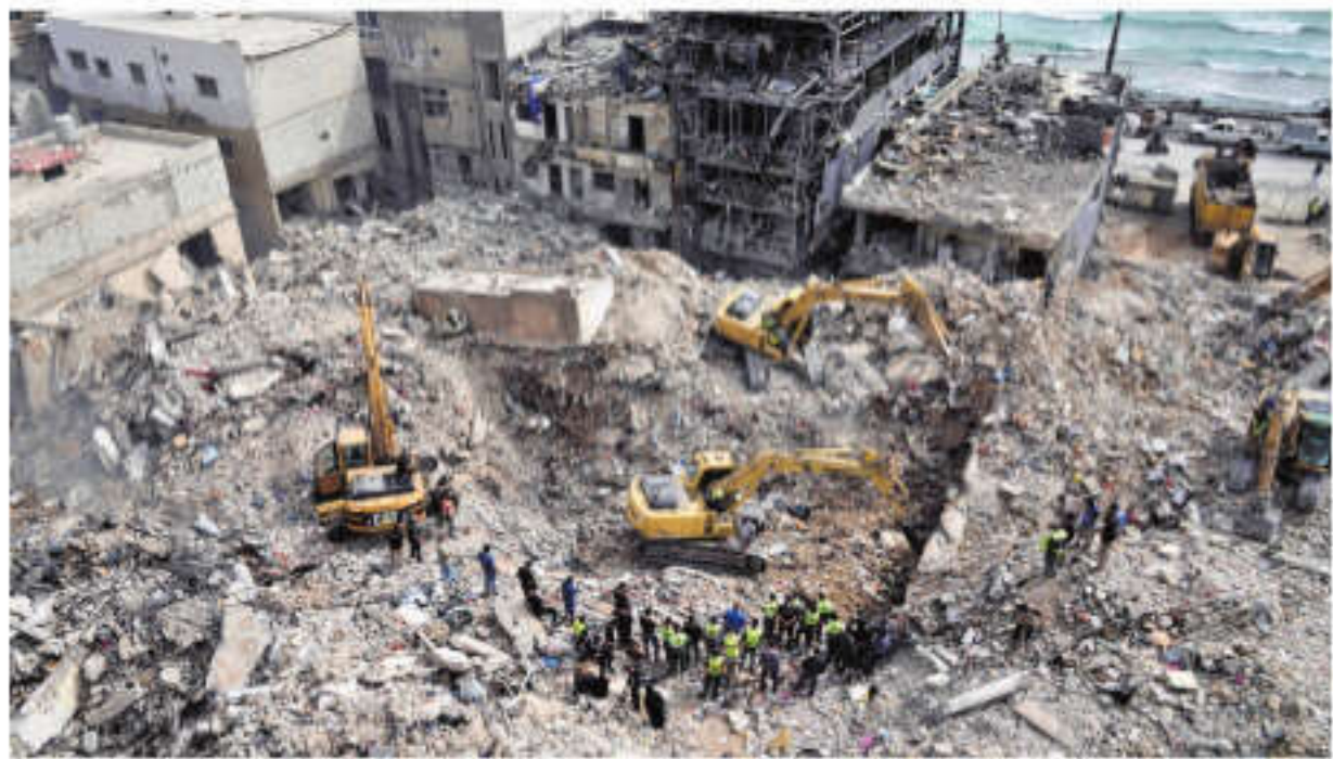
Excavators remove rubble from buildings destroyed in Israeli airstrikes on Thursday as rescuers search for victims in the city of Tyre, southern Lebanon | AP
